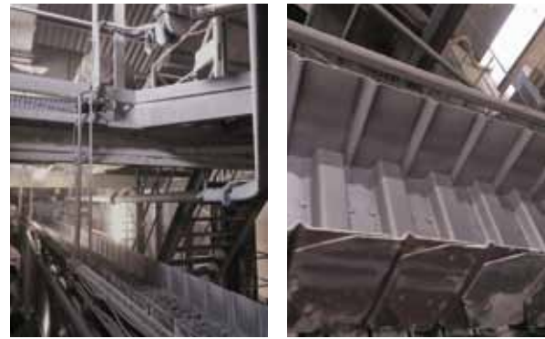
Figure 4: Bulkscan® sensor over inclined pan conveyor for clinker transport (left) and an empty clinker cooler pan conveyor
